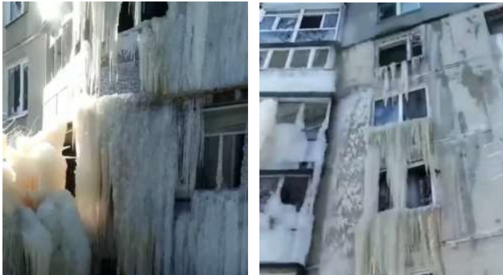
Fig. 1. Heating system violation.
